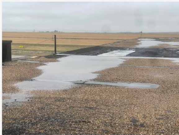
Significant water ponding on roof
